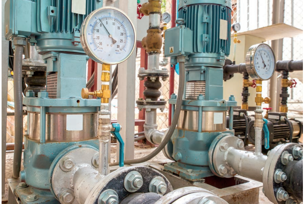
Always check for corrosion and erosion.
